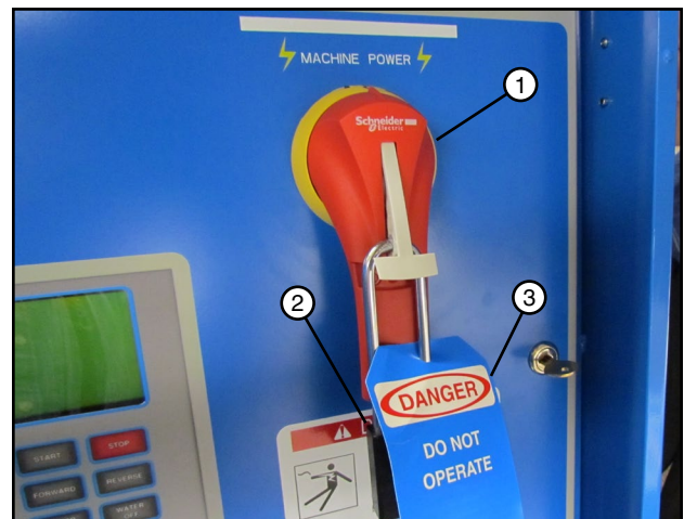
Figure 29-2 1. Main Disconnect 2. Lock 3. Blue Tag
