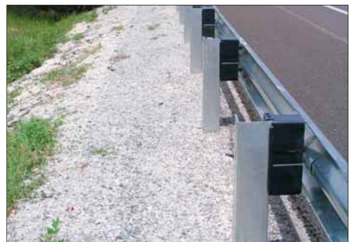
Steel block failure
