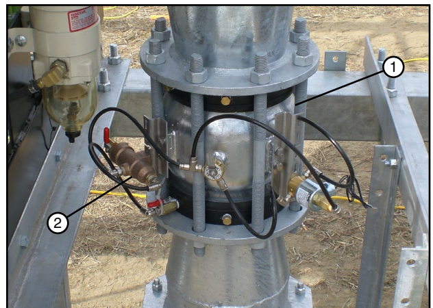
Figure 91-4 1. Water Shut Off Valve 2. External Filter
