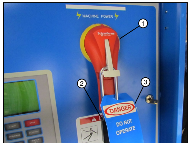
Figure 91-2 1. Main Disconnect 2. Lock 3. Blue OSHA Tag
