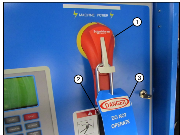
Figure 105-2 1. Main Disconnect 2. Lock 3. Blue OSHA Tag
