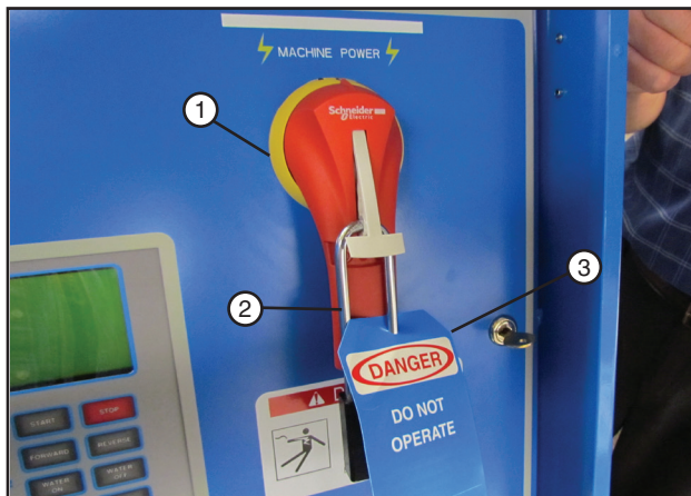
Figure 90-2 1. Main Disconnect 2. Lock 3. Blue OSHA Tag
