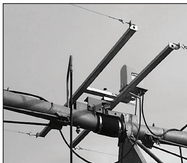
Figure 27-3 Pivot Floating Alignment - Most Sensitive
