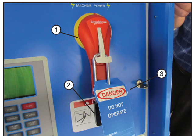
Figure 103-2 1. Main Disconnect 2. Lock 3. Blue OSHA Tag
