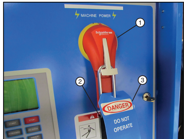
Figure 105-2 1. Main Disconnect 2. Lock 3. Blue OSHA Tag
